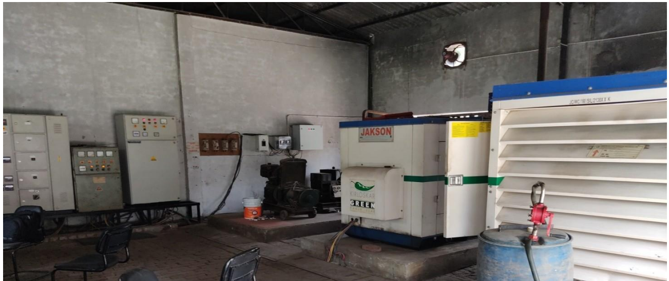
Electricity Generator Room
