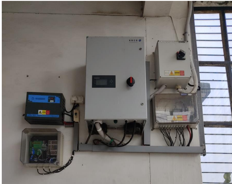
Solar Inverter and Metering
